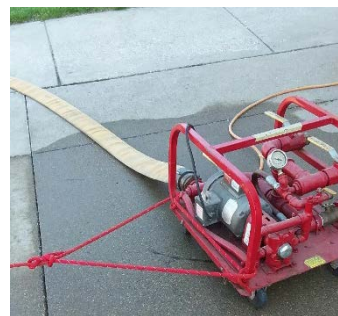
Test pump used during the rupture
