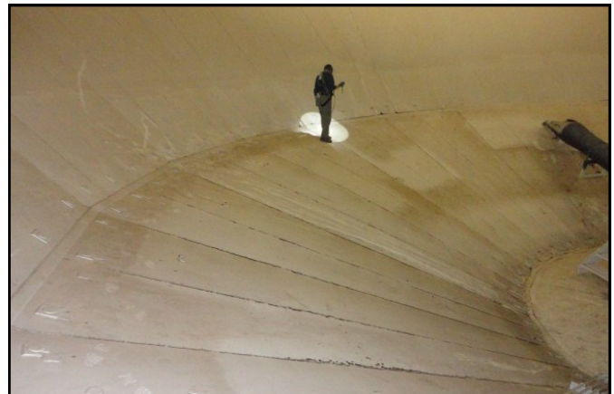
A Navy-contracted worker inspects the bottom of Tank 5 at Red Hill Bulk Fuel storage facility.
