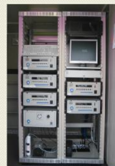
CAM system at the Support Site in Gricignano.
